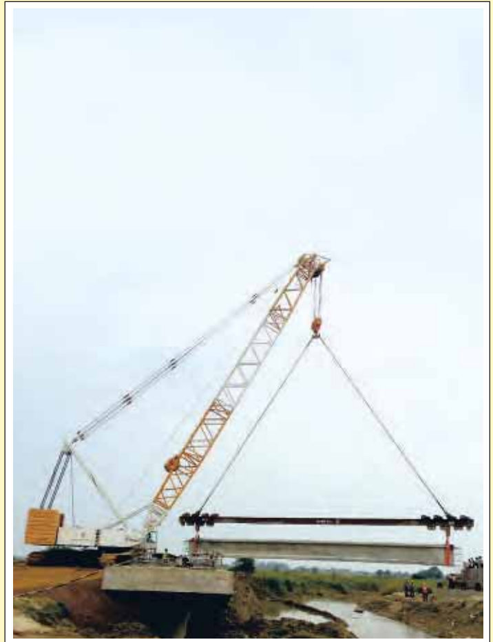
DEMAG CC 2400 (Capacity 450 MT) Crawler Crane, main boom 36M erecting Bridge Girder 80 MT at Afcons Infrastructure Limited site at Etawah, Uttar Pradesh
