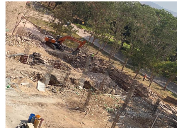
Baghouse and MCC Room
