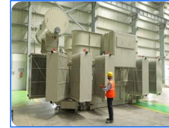
Oil Filled Reactors
