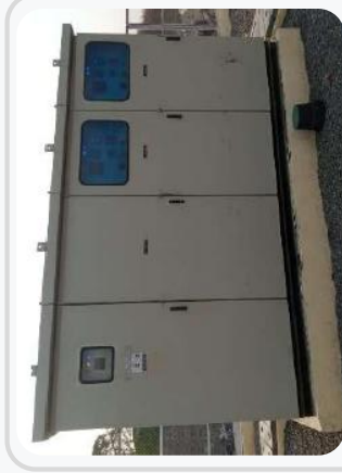
33kV RMG Panel
