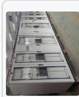
Power Control Centres (PCC) Panels
