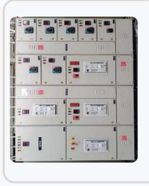
Intelligent Motor Control Centre (IMCC) Panel
