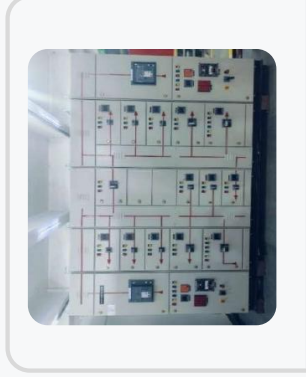
Motor Control Centres (MCC) Panel
