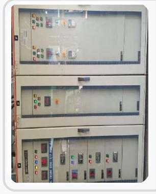
Variable Frequency Drive (VFD) Panel
