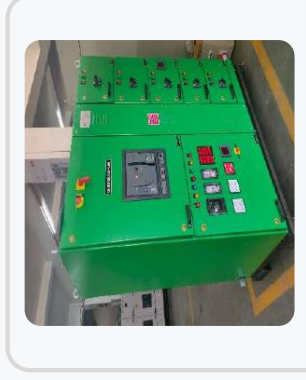
DG Synchronizing & Load Sharing Panels
