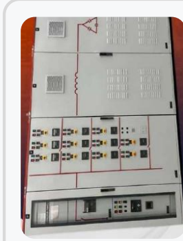
Automatic Power Factor Correction (APFC) Panel
