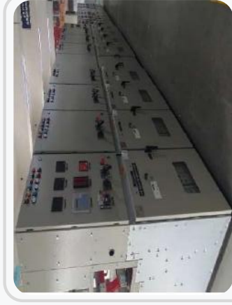
11kV DG Synchronizing & Load Sharing Panels
