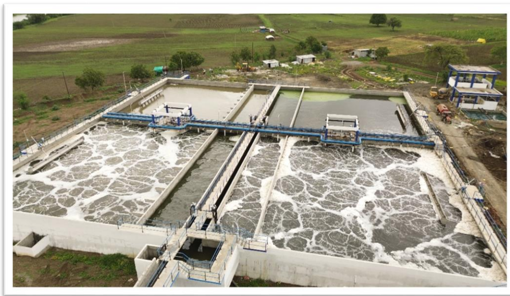
32 MLD STP Plant at Latur, Maharashtra
